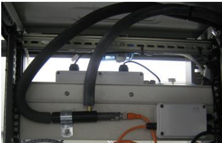
Figure 158 – Example of installed CO 2 Sensor
