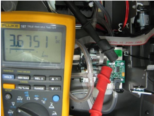
Figure 63 – Typical Test Point Reading of Manifold Pressure Sensor
