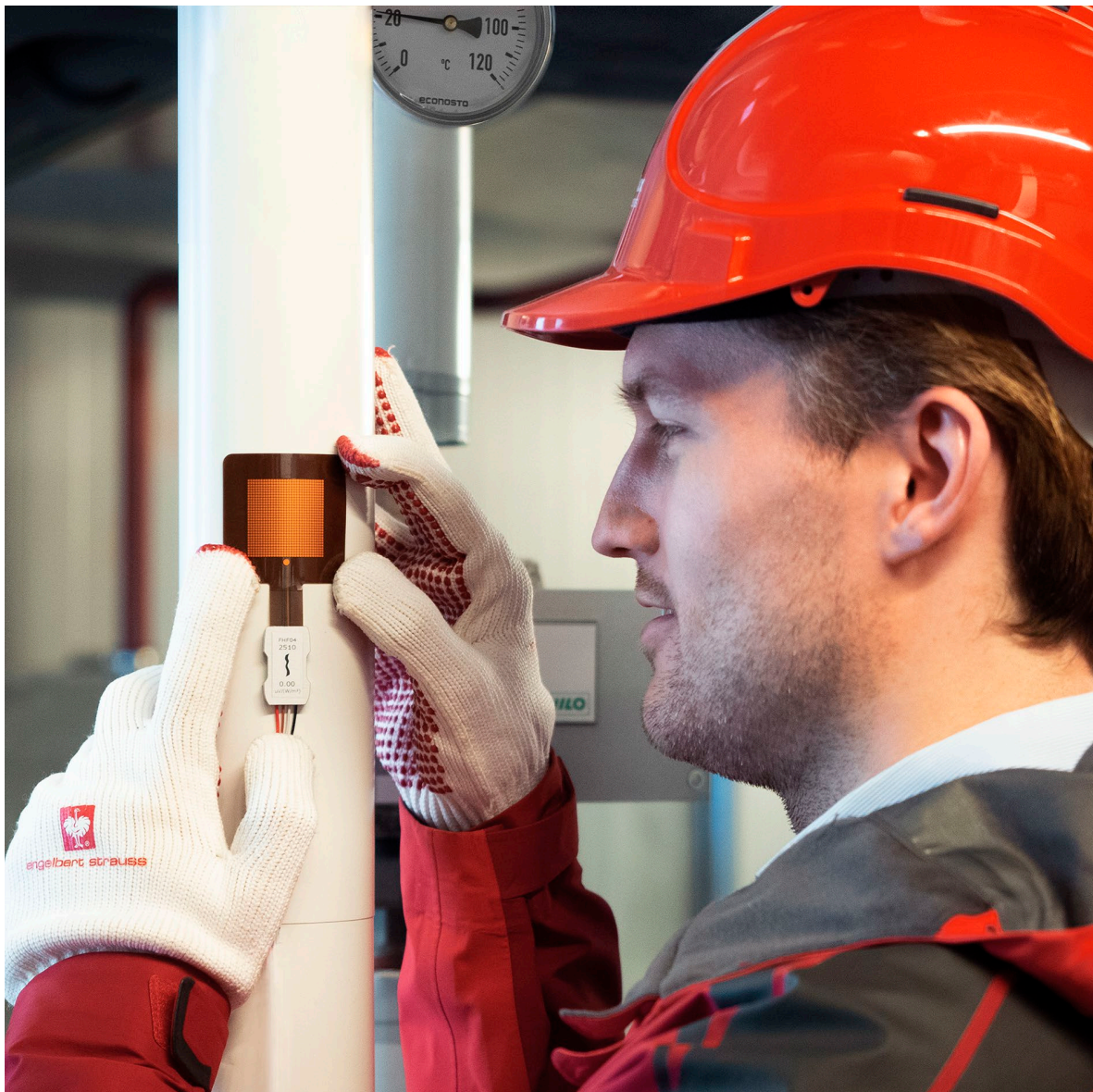
Figure 4.1.1 Example of an FHF04SC foil heat flux sensor being installed for measurement on an industrial pipe. The sensor is mounted on a well-prepared curved surface.
