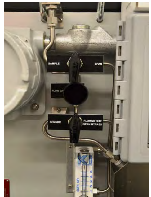
Picture View of Two Valve Configuration
